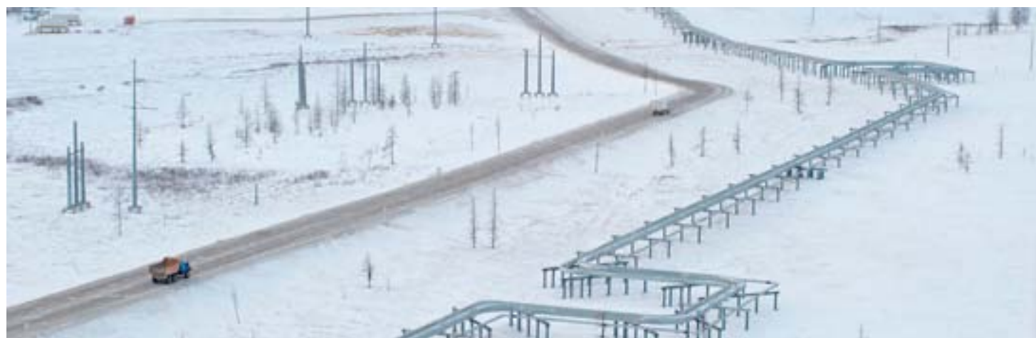
Vankorneft's pipeline system.
